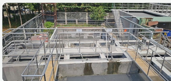
Wastewater Treatment Facilities
